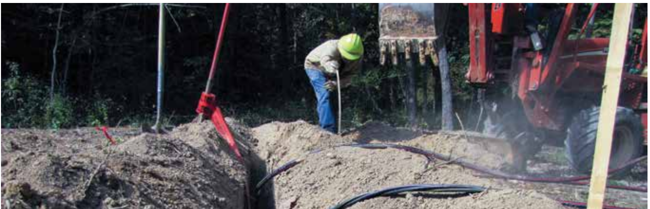
Line Foreman Bill Hart determines the site of a transformer pad as he oversees the underground project.
