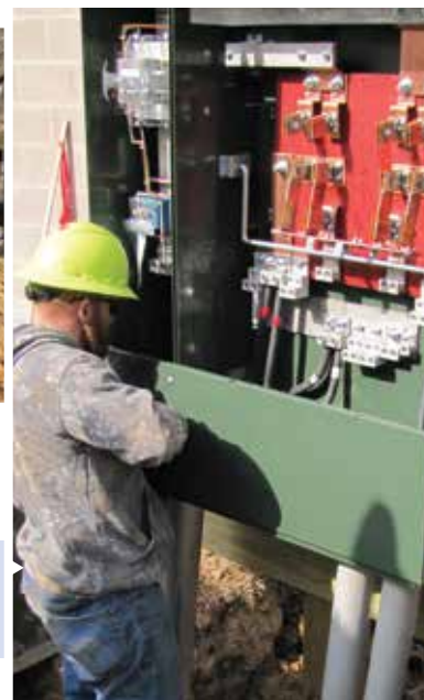
Intern Matt Evans removes cover panel from an 800-amp cabinet.
