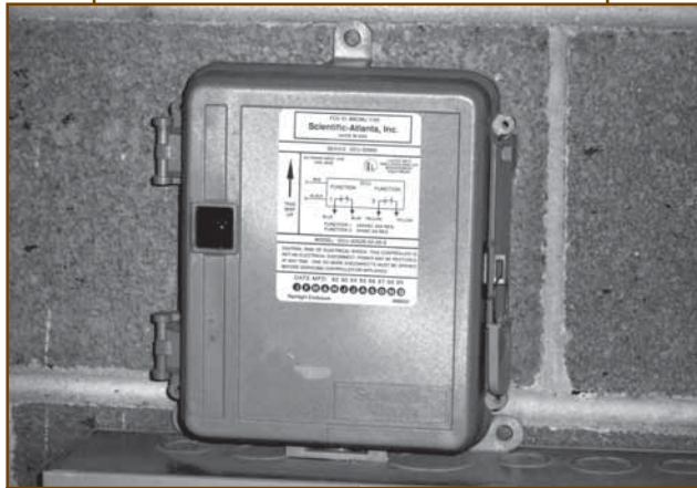
One of the Peak Switch boxes used by RECC
