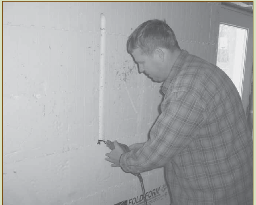
Moe Gibbs cuts a channel in the foam insulation board with a “hot knife” tool for installation of electric wiring circuits in a basement wall.
