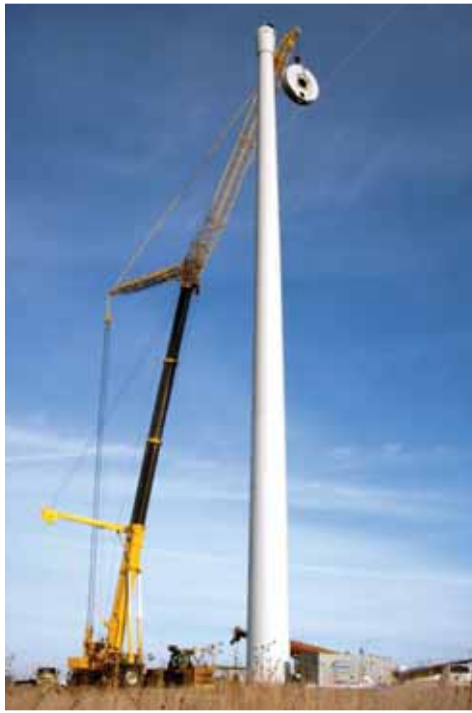
A huge crane, with the help of a “small” crane, lifted the three-tower section into place, then placed the nacelle on top that would hold the generator and blades.
