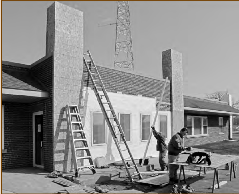
A stucco-like finish will be applied to the center section of the new façade when warmer temperatures return.
