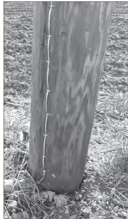
Copper ground wires are installed on electric poles to provide safety protection and proper operation of protection equipment.
