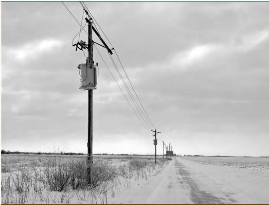
A stretch of line north of the Kincaid Power Plant had 20 broken cross arms, which kept power off for members in the New City area overnight on Tuesday, Feb. 2.
