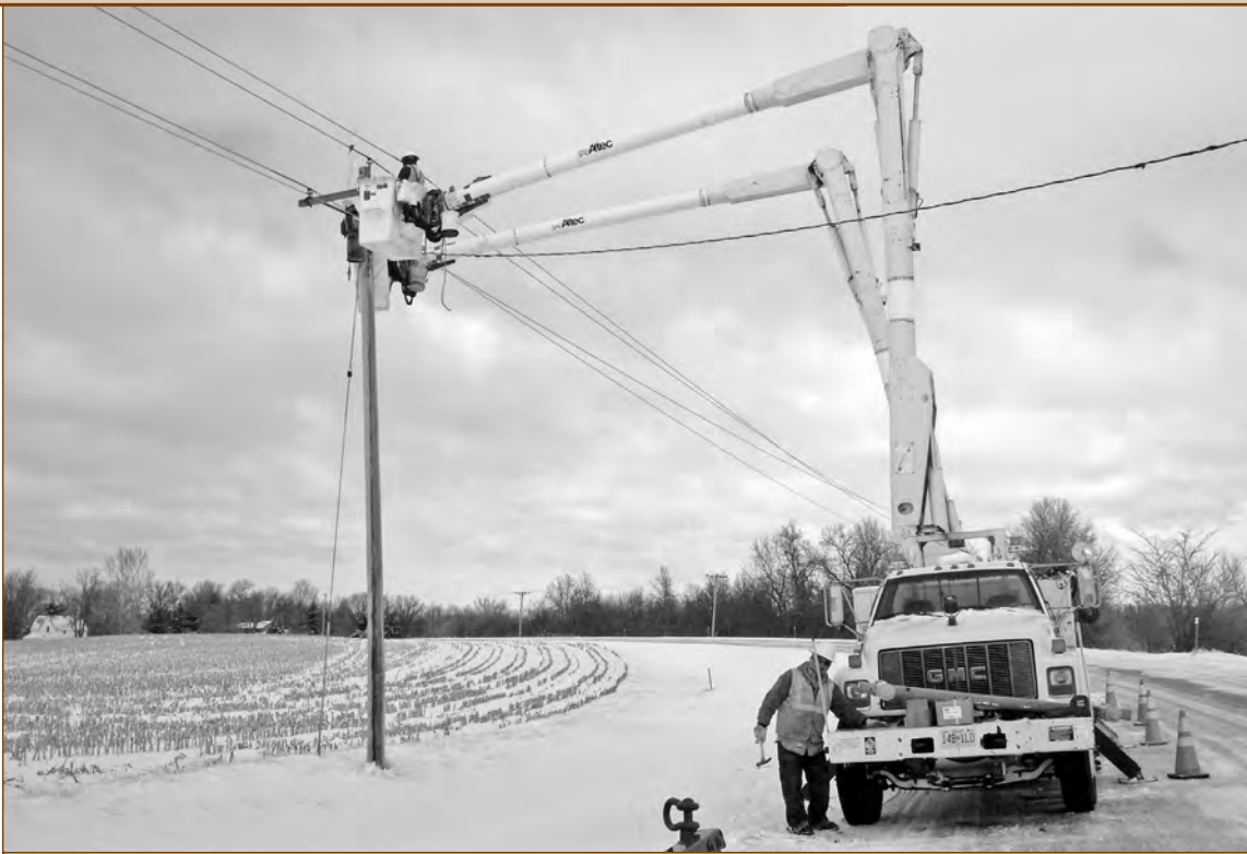
Extra crews from Croft Electrical Contractors helped make repairs after the ice and snow storm, and clear weather on Wednesday made work much easier than in the blowing snow on Tuesday.
