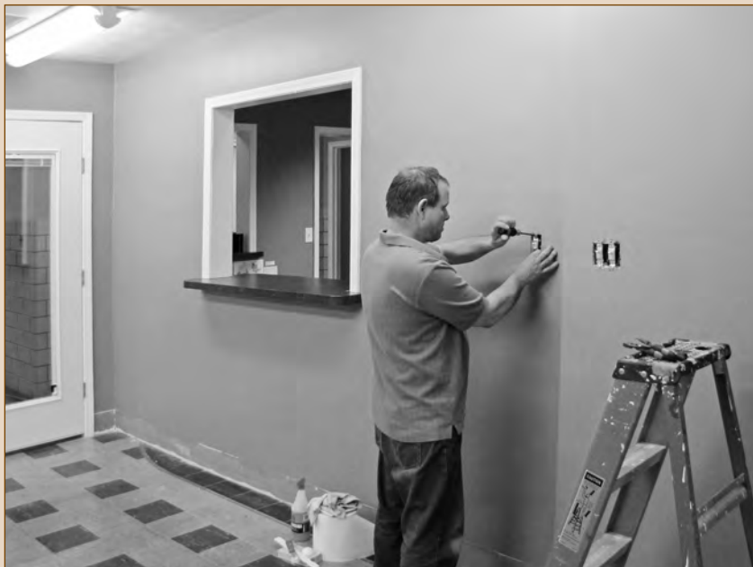
Custodian Stefan Sporer, one of the co-op employees who has done the painting and finish work inside, replaces a switch near the new service window in the front lobby.
