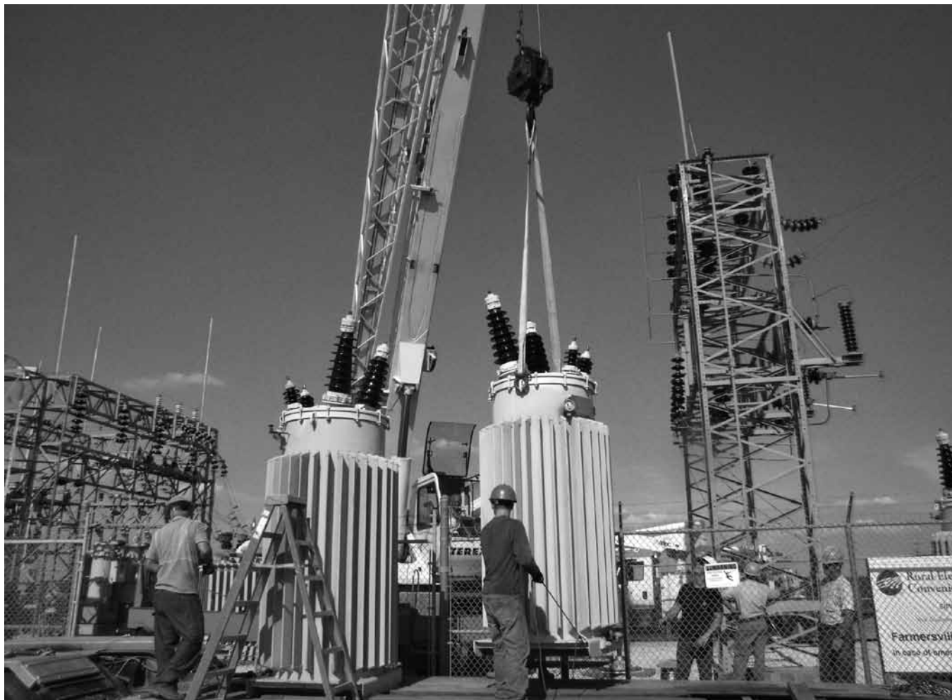
One of the six smaller transformers is lifted out of the Farmersville substation after the failure of one transformer on July 1. A single 5000-KVA transformer was installed, doubling the capacity of the substation.
